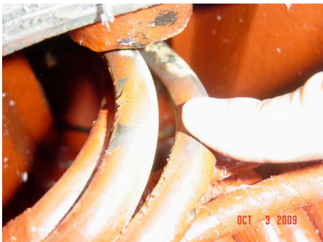
Fig. 10 Defects causing PDs of Motor #4
