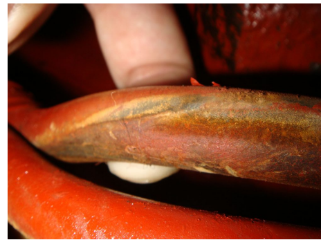
Fig. 11 Defects causing PDs of Motor #5
